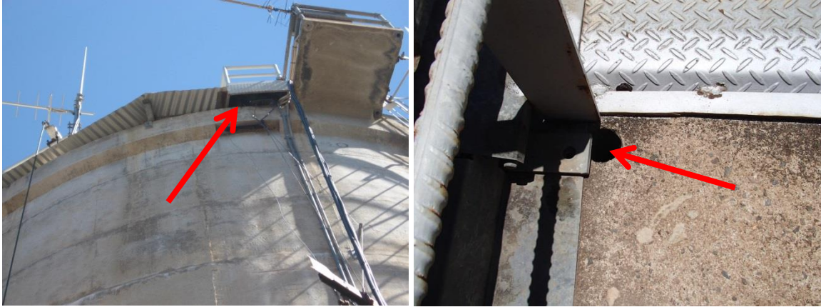
Figure 5 Reservoir images, with arrows showing some of the vermin entry points
