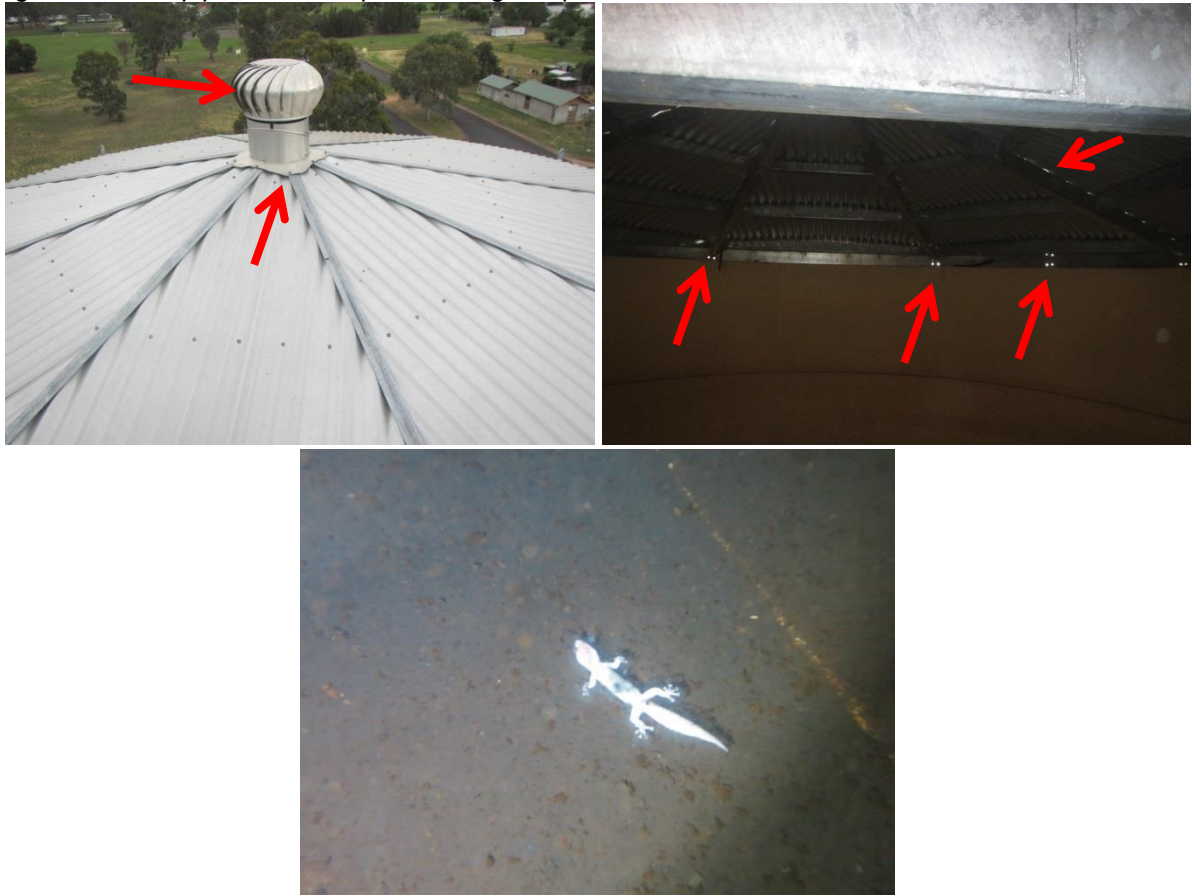
Figure 34 Standpipe Reservoir potential ingress points, and evidence of contamination
