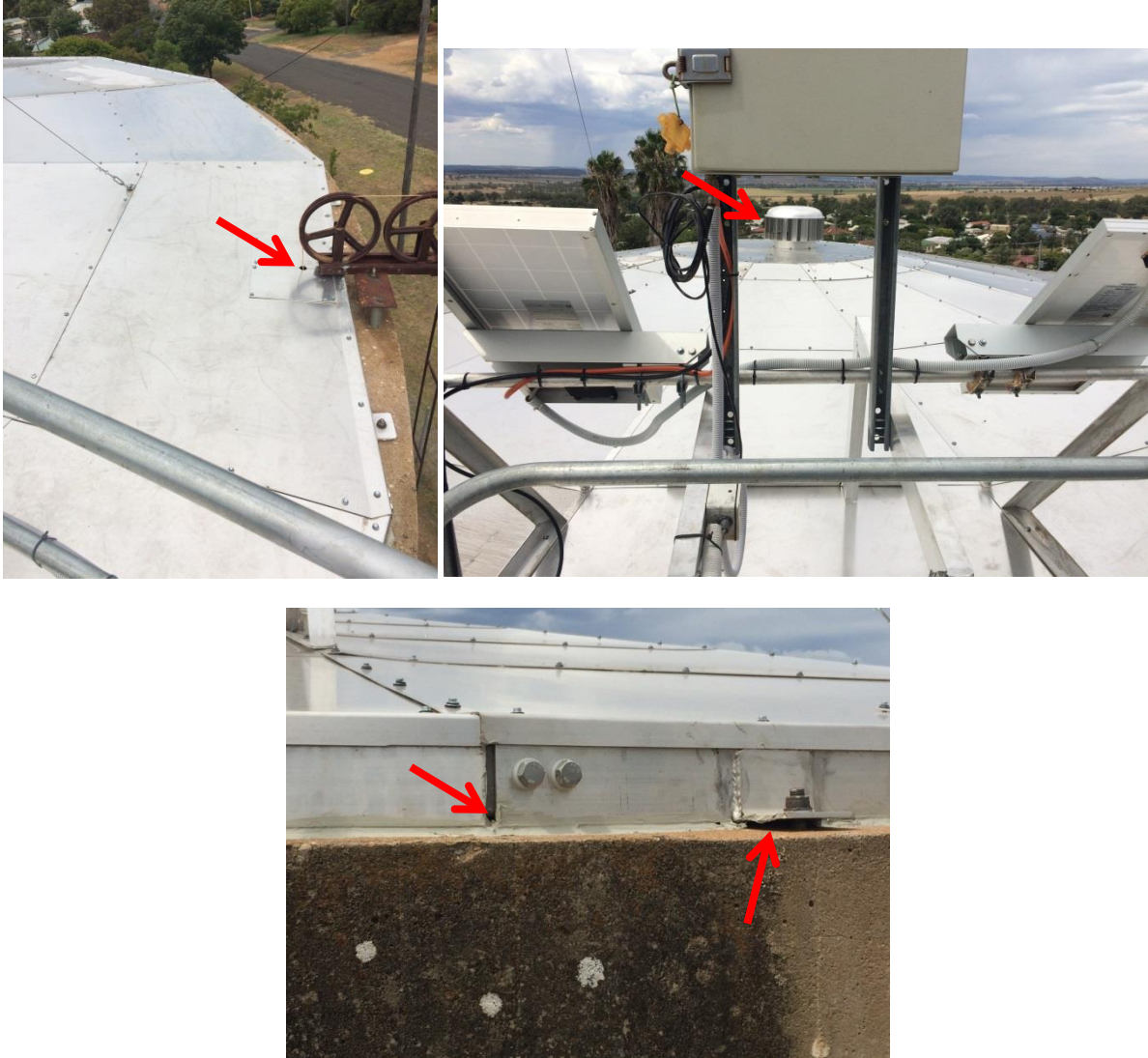
Figure 28 New Roof on Bullinda St Reservoir - some potential access points remain
