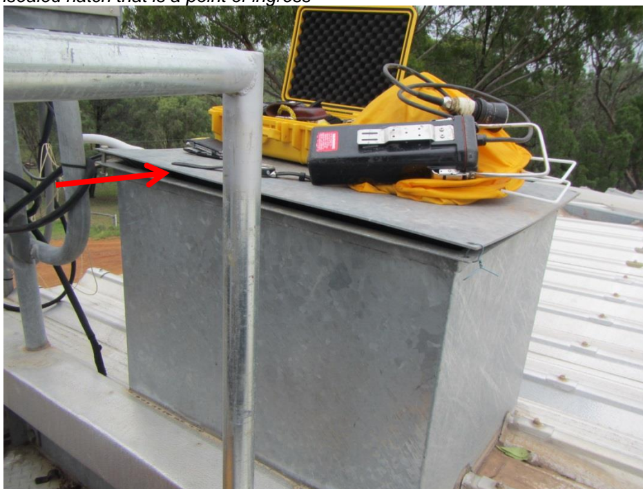
Figure 9 Unsealed hatch that is a point of ingress
