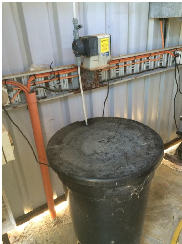
Figure 11 Chlorine dosing shed, Bugaldie
