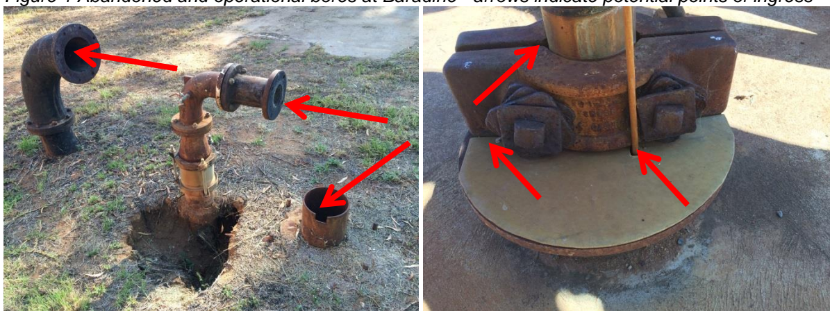
Figure 1 Abandoned and operational bores at Baradine - arrows indicate potential points of ingress
