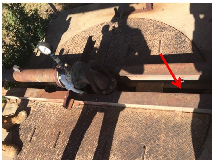
Figure 15 Bore 2 - well style, and unsecured from vermin access
