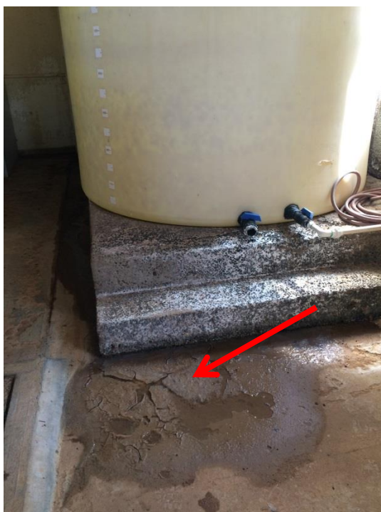
Figure 2 Chemical tank showing evidence of a spill immediately adjacent to clear water tank hatch.
