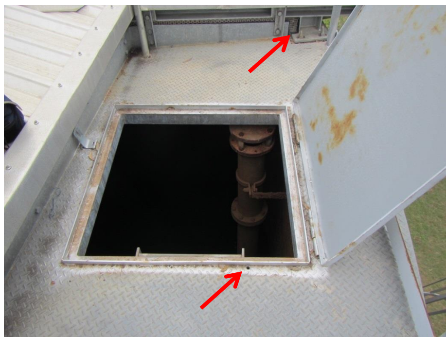
Figure 7 Possible ingress points near access hatch, Binnaway reservoir
