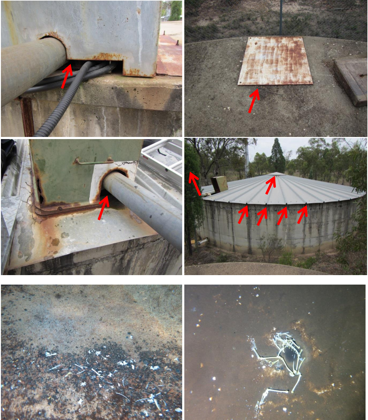
Figure 35 Coolabah Reservoirs 1-3 points of ingress and contamination evidence (animal bones)
